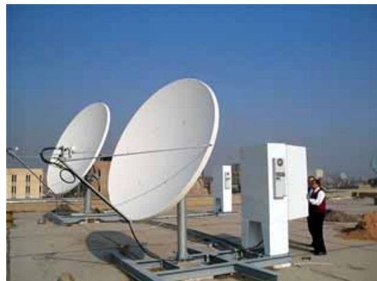
VSATs Installed in Baghdad
