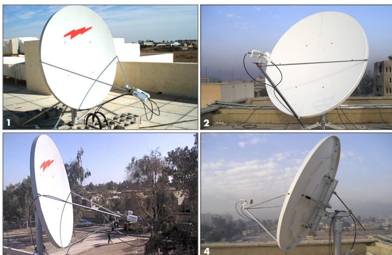
1, 2, 3, 4) Some VSAT systems installed in Baghdad and other provinces
